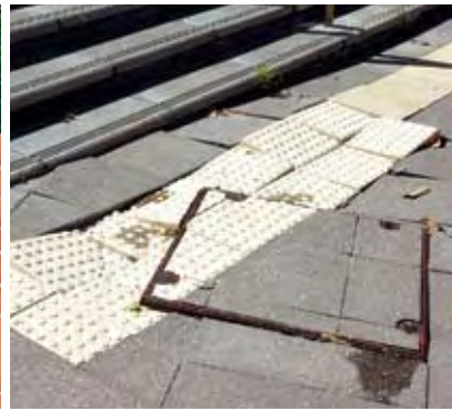
FIGURE 138 Subsidence of paving above inadequately backfilled and compacted service trench
