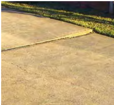
FIGURE 139 Stepping at joint due to settlement of subgrade
