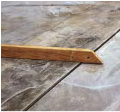
FIGURE 190 Curled slab edge of industrial pavement
