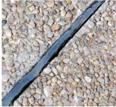
FIGURE 179 Loss of adhesion due to inadequate preparation
