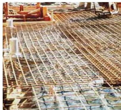
FIGURE 141 SL81 mesh used to control cracking where the surface of the slab will be exposed (polished concrete finish)
