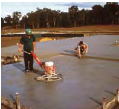
FIGURE 32 Power trowelling used for large areas and hand trowelling for corners and edges
