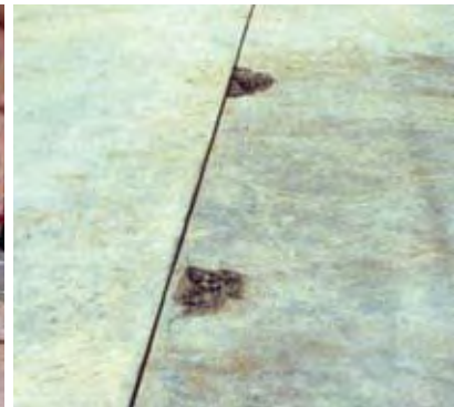
FIGURE 193 Cracking and spalling at anchorages of post-tensioned warehouse slab due to premature stressing of the slab tendons
