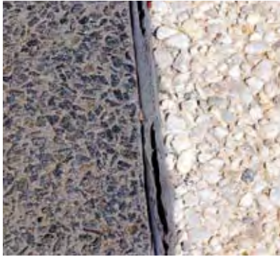
FIGURE 178 Expansion capacity of sealant exceeded
